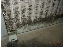
Microbial growth on the Evaporator coil prior to cleaning
